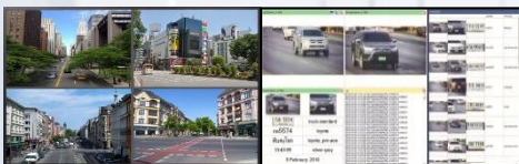
Monitor CCTV and License Plate
