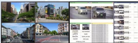
Monitor CCTV and License Plate
