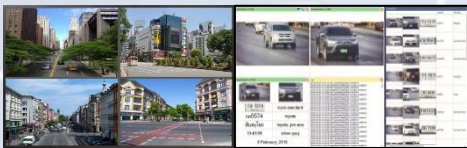
Monitor CCTV and License Plate
