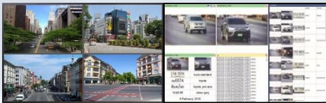
Monitor CCTV and License Plate
