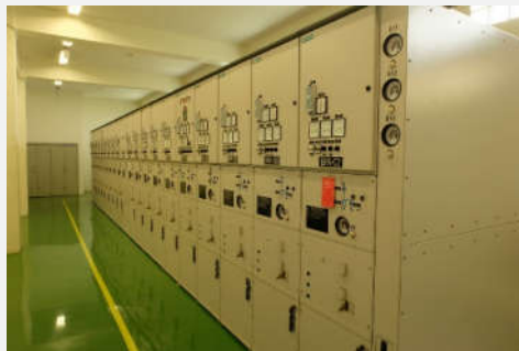
Medium Voltage Switchgear
